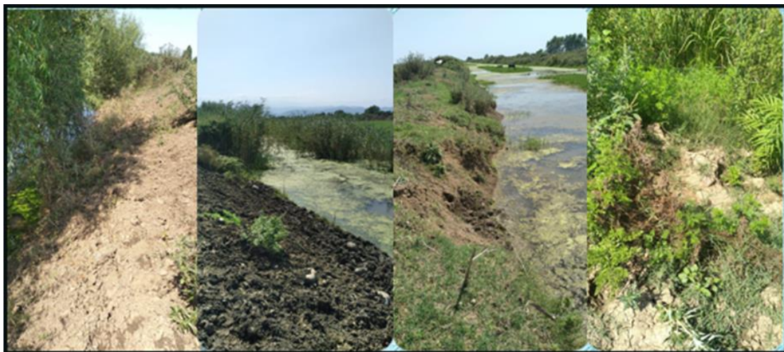
Figure 9. Washout, erosion, landslides and collapse of collector slopes
